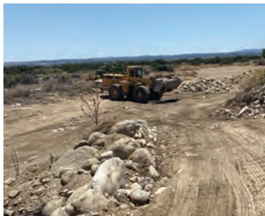
Recharge basins at the Santa Ana River Groundwater Recharge Facility require regular maintenance to remove trash and unwanted vegetation. Photo Credit: SBVWCD
