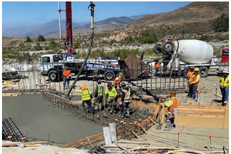
Construction underway at the Santa Ana River's Mill Creek diversion percolation basins. Photo Credit: SBVWCD.
